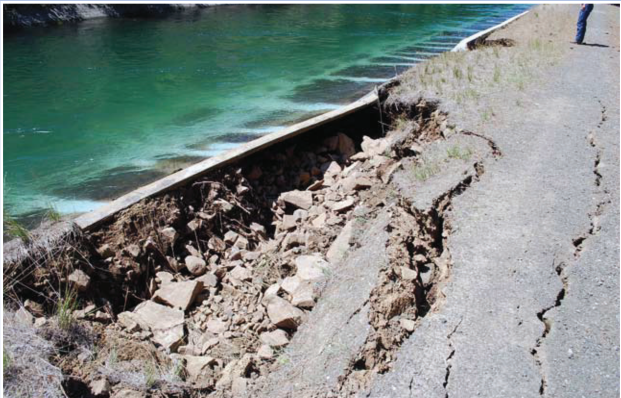
Damage to the canal bank on KRD's Main Canal.
